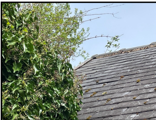
Plate 4 Occasional gaps exist under roof slates and ridge tiles
