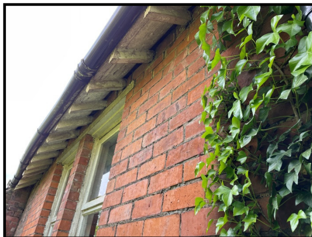
Plate 3 Gaps under eaves on east elevation
