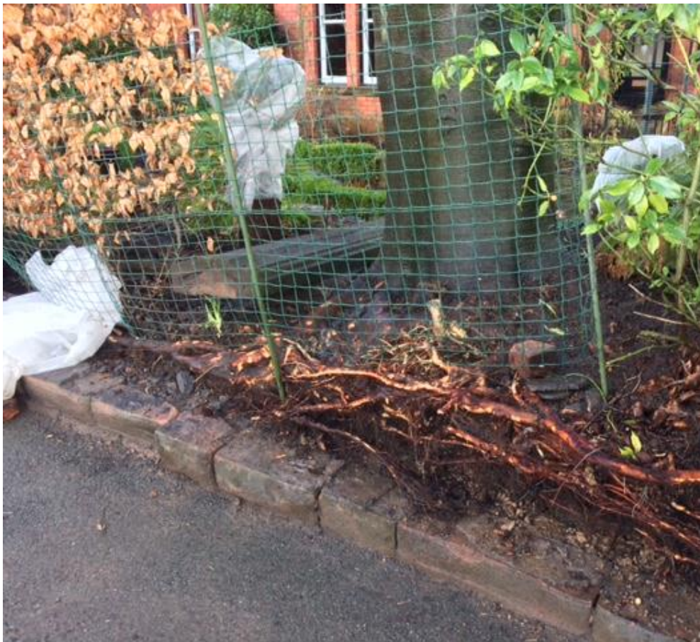
Image 2 - Wall has been dismantled and revealed extent of stunted roots which are recommended to be removed
