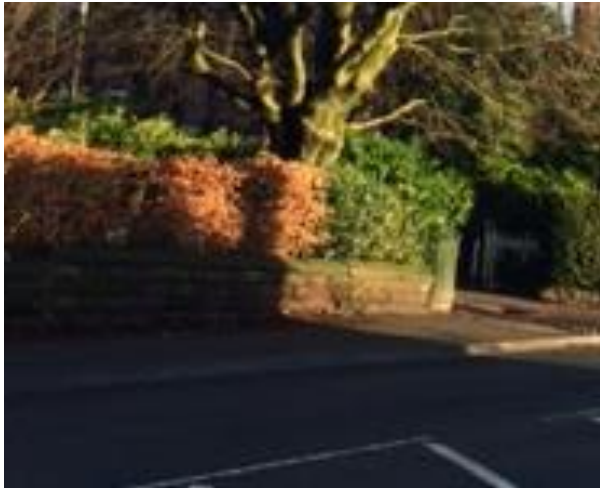
Image 1 - wall which was becoming dangerous due to risk of collapse onto pavement
