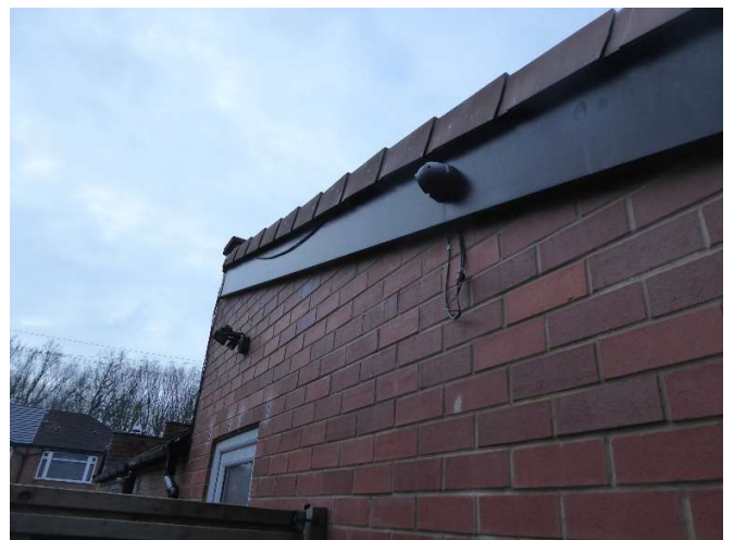
East side elevation showing fascia with minor gaps at low level.
